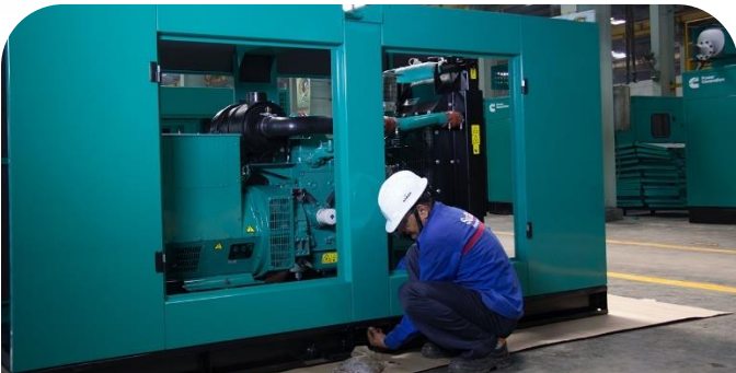
DG & Repair Maintenance
