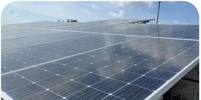
Solar EPC Excellence
