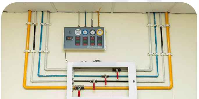
Medical Gas Pipelines
