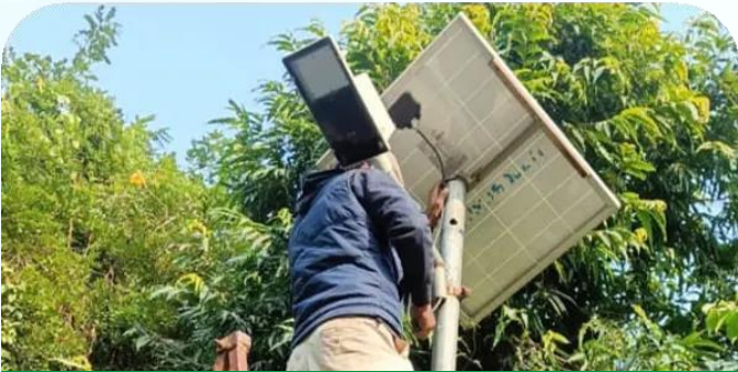
Solar Street Lights
