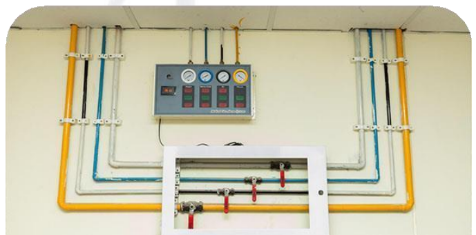
Medical Gas Pipelines
